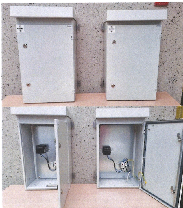
Figure 1. Electrical boxes delivered for testing (daytime view, before measurements, outside the building).
